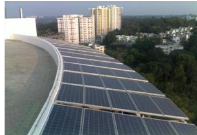
25kW Solar Photovoltaic Arrays
