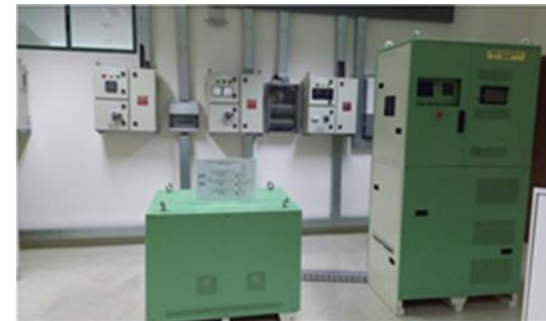
Power Conditioning Unit- Solar
