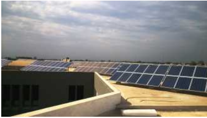
Fig. 1. Solar Photovoltaic System
